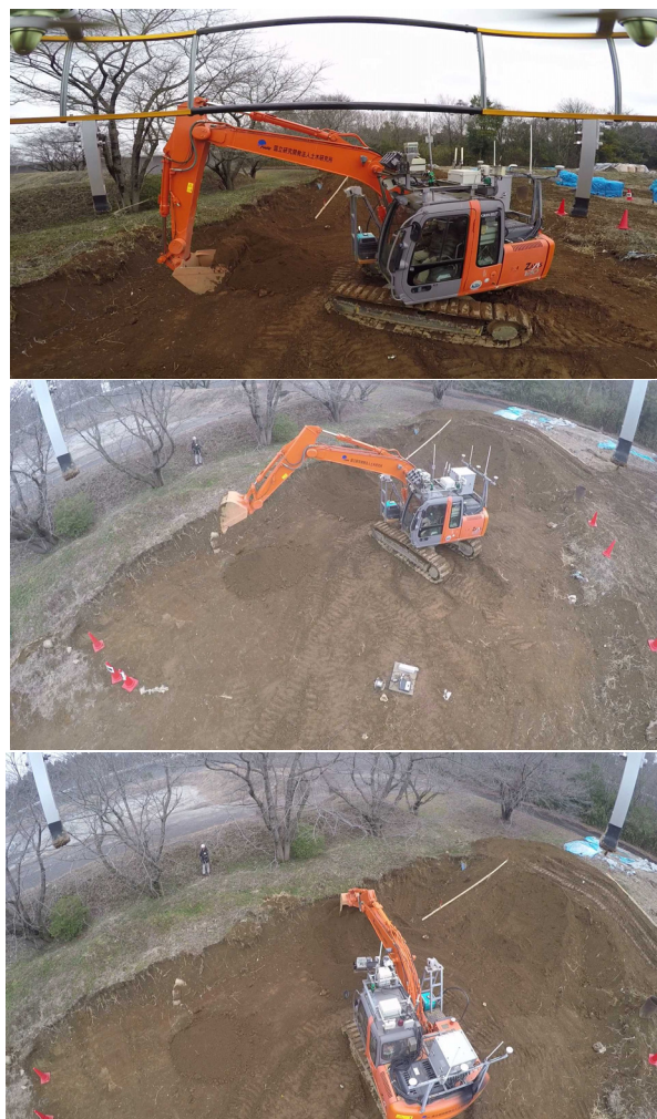
Fig.6 Visual information obtained by GoPro. (1) Left side, very close, about 2.5m height from the ground. (2) Left side, a little bit high position: about 6.0 m height from the ground. (3) Back side, about 6.0 m height from the ground.
